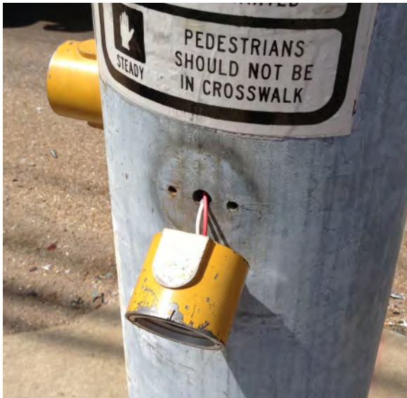
Push-buttons will require regular inspection
