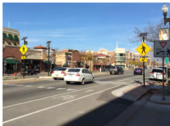
Rapid Rectangular Flashing Beacons (RRFBs) in Ogden, Utah
